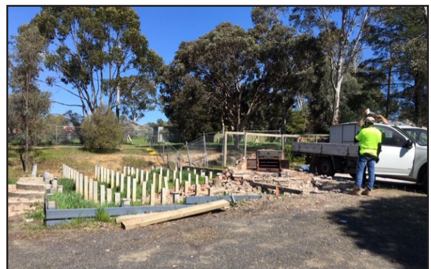
Demolition of the last remaining structure of the Tallarook Mechanics' Institute - the chimney (Photo: Libby Webster)
