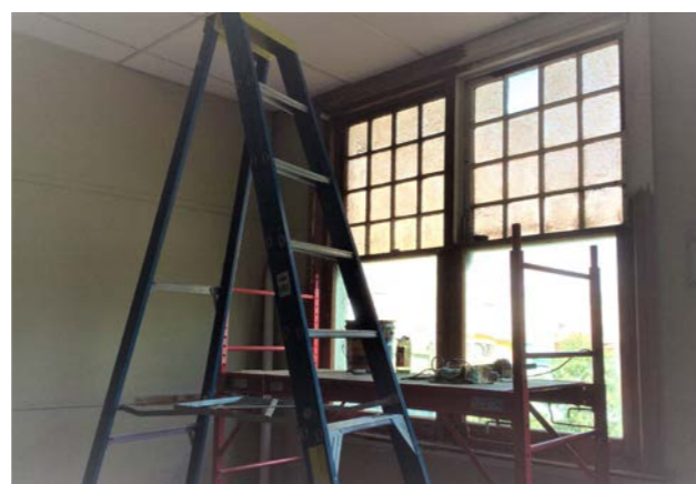
Ladders and scaffold in place in the Snooker and Billiards Room during recent renovations.
