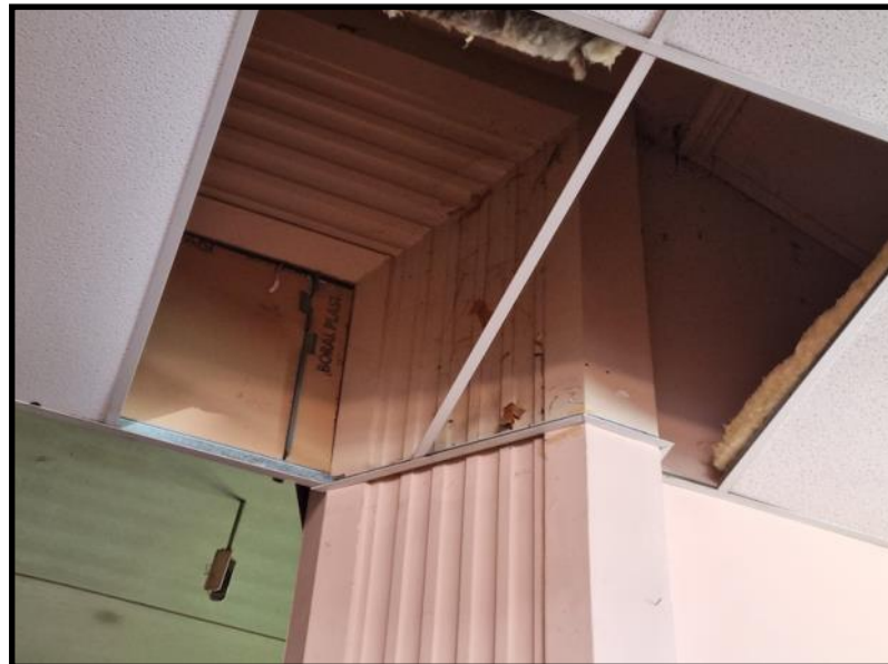
The c.1933 Proscenium Arch and ornate plaster cornice were uncovered during renovation works.
